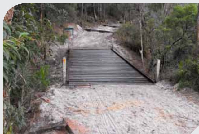
Frankie's Gulch Bridge before and after (Source: Department of Environment and Resource Management).
