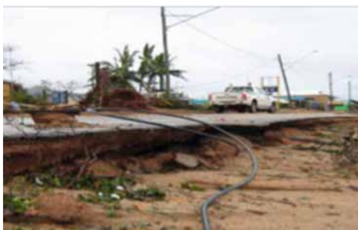
Damage to Bruce Highway during the summer of 2010-11 (Source: Department of Transport and Main Roads).
