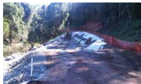
Amamoor Creek Road (Source: Queensland Reconstruction Authority).
