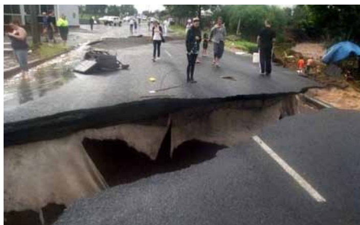
Flash flooding leaves a hole in Jellicoe Street where it crosses Gowrie Creek (Source: Getty Images).
