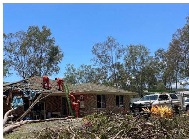
Figure 36. SES teams were deployed from across the country to support the storm relief effort. Image: ABC News
